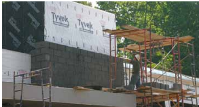
After a wet winter and spring that delayed some construction, the Literacy Building is taking shape.
