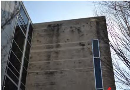
Water stains on facade
