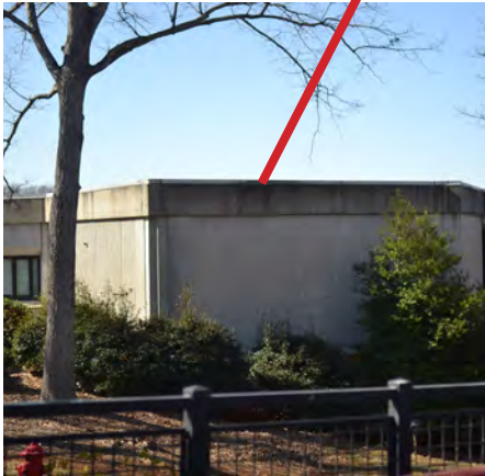
Water stains from roof
