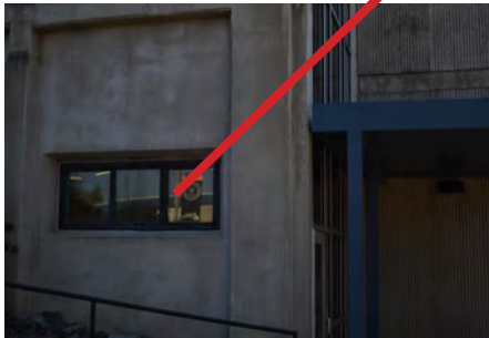
Windows to be replaced
