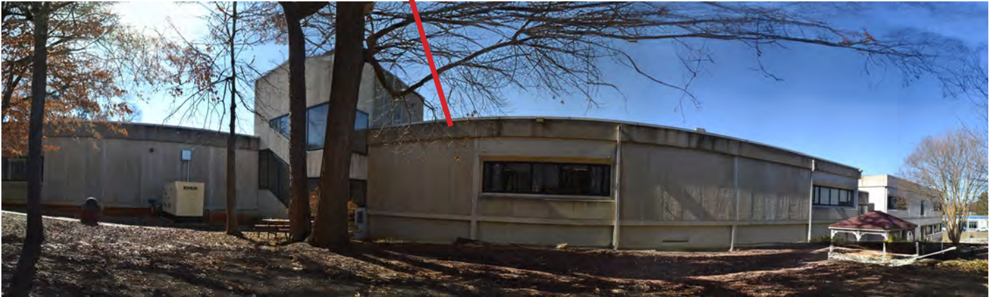
Water stains from roof
