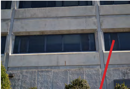
Concrete material stains
