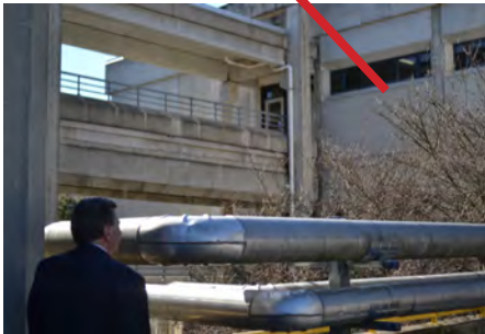
Concrete material stains
