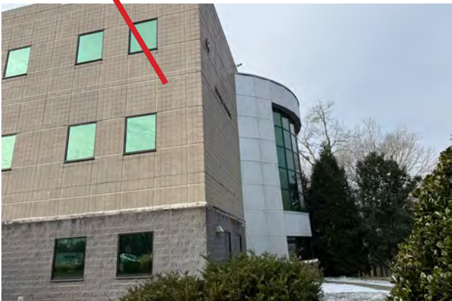
Facade improvements required
