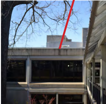
Water stains from roof
