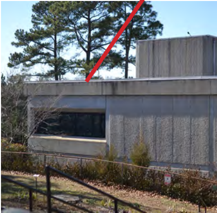
Water stains from roof
