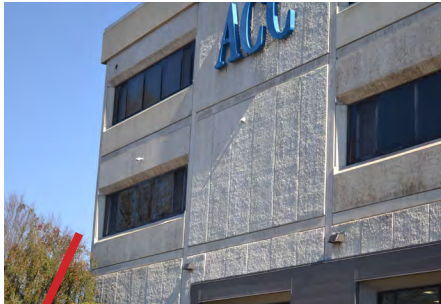
Concrete material stains
